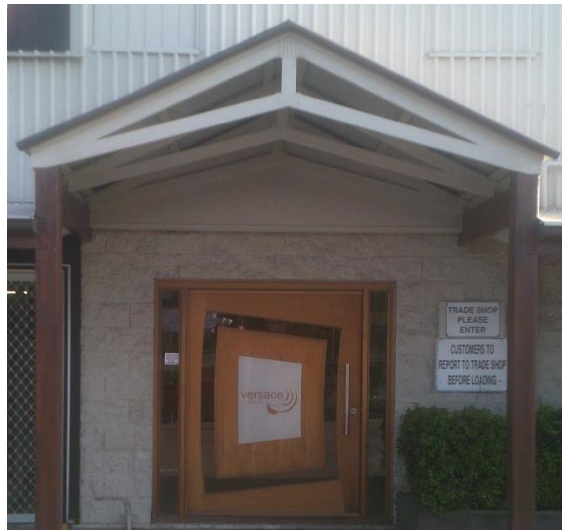
SADLY THE ENTRY DOOR DIDN'T MEET CODE
